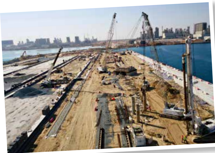
Oil and gas terminal Borouge 3, Al Ruwais, UAE
