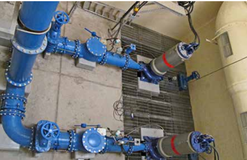
Water pumping stations, Abu Dhabi, UAE
